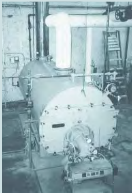
This fuel oil boiler used to heat one of the Darby schools and now serves as backup to the new three-school woodchip system, providing complete protection in case of any situation that may arise.
